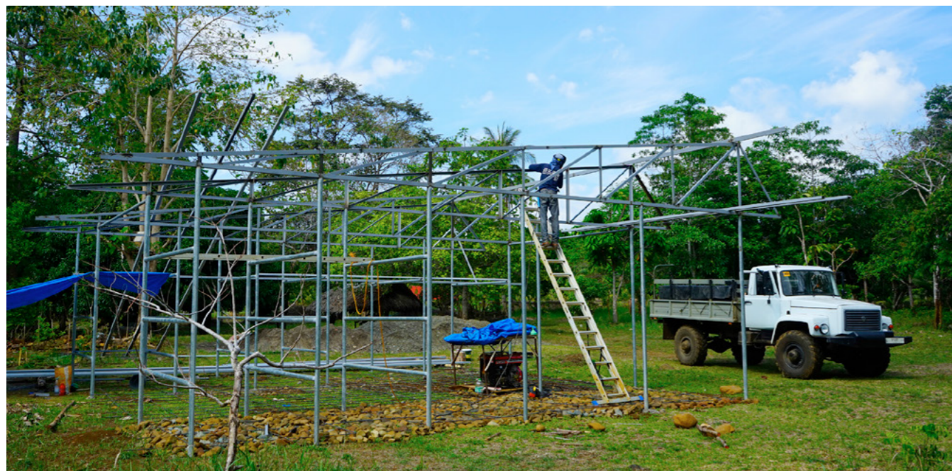
Storage and garage construction. Our Apprentices get the opportunity to practice their newly acquired skills.
